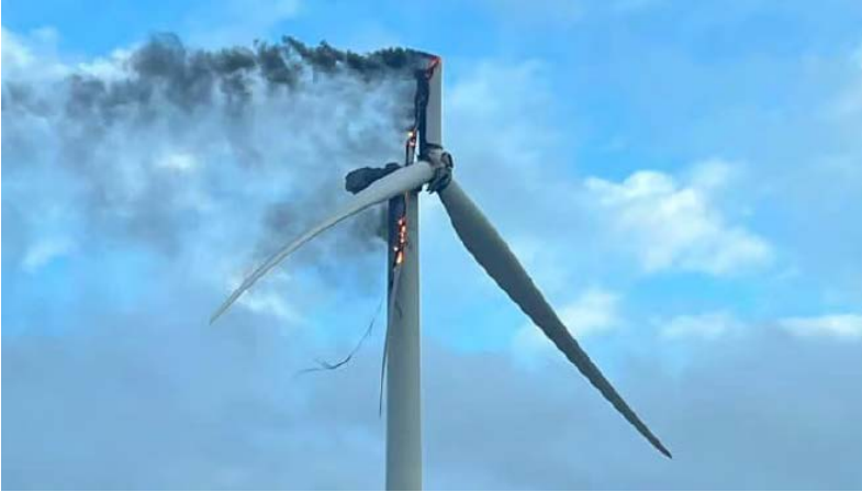
Goulburn Wind Turbine Fire January 2023
